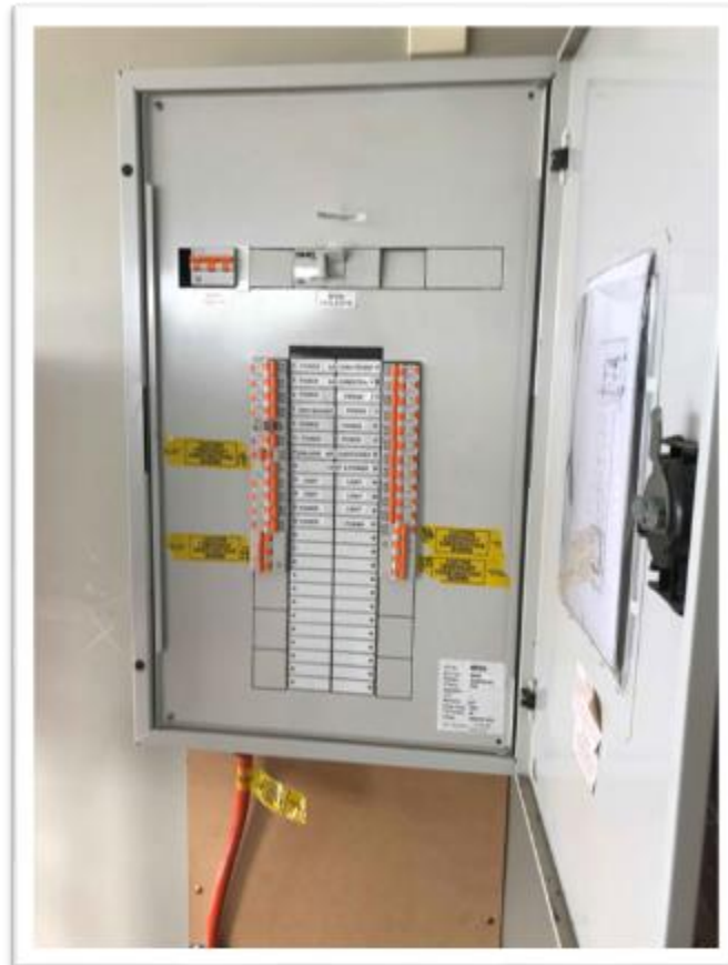
New Distribution Board with 3 phase supply
